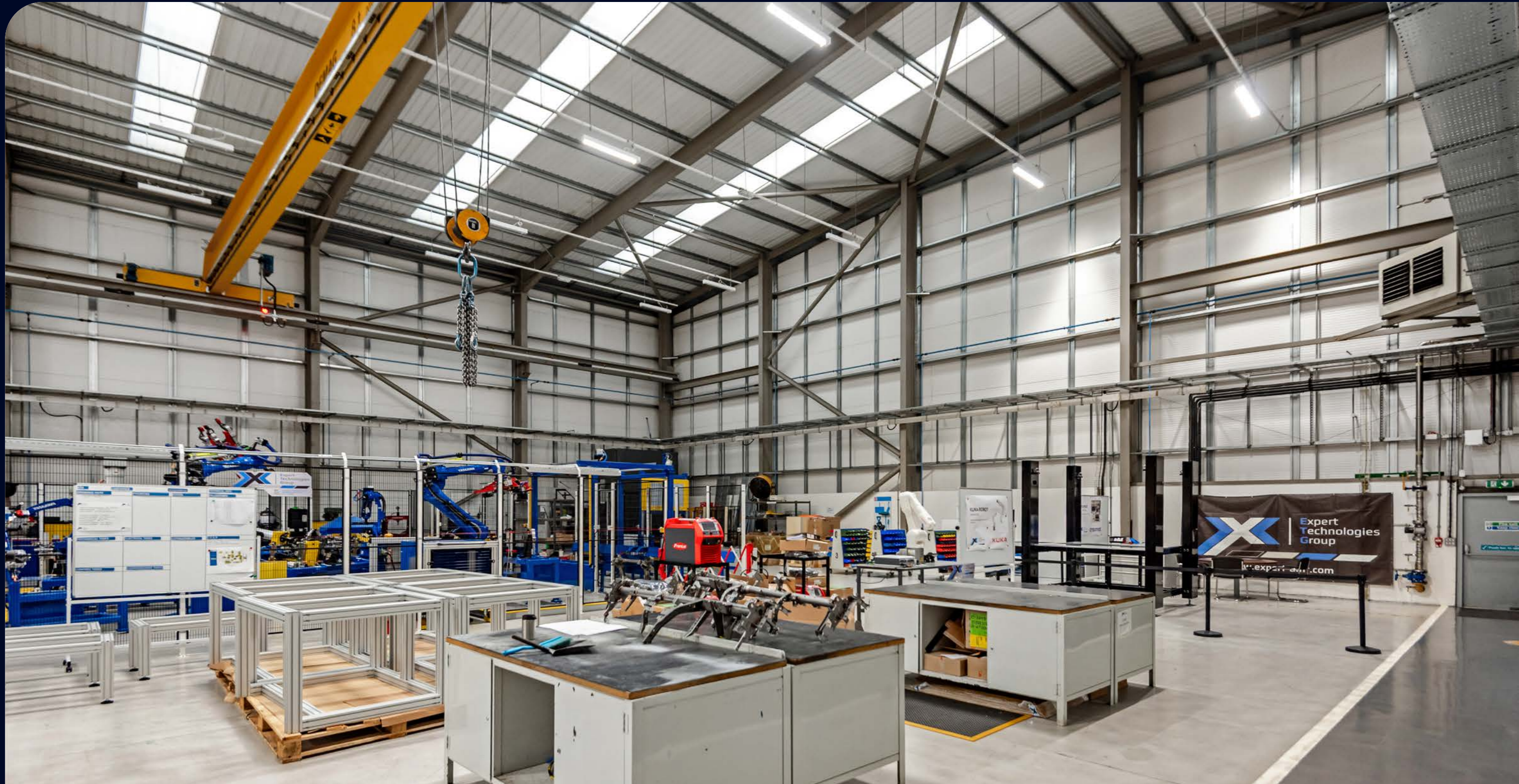
Warehouse with two 8 tonne gantry cranes within the warehouse which are 7m to underside of beam
